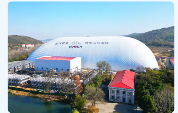
Carbon dioxide Energy Storage Demonstration System
