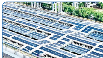
Centralized grid connection of three new photovoltaic power stations
