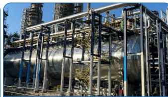
Successful commissioning of tertiary electric desalting revamp project
