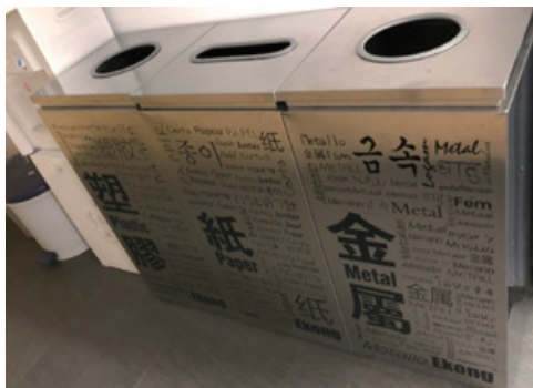
Waste categorisation: installation of different types of waste collection bins 垃圾分類：設置不同類別收垃圾箱
