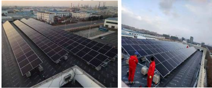
▲ Solar PV Power Generation on the Roof of the Pipe Fittings Center
