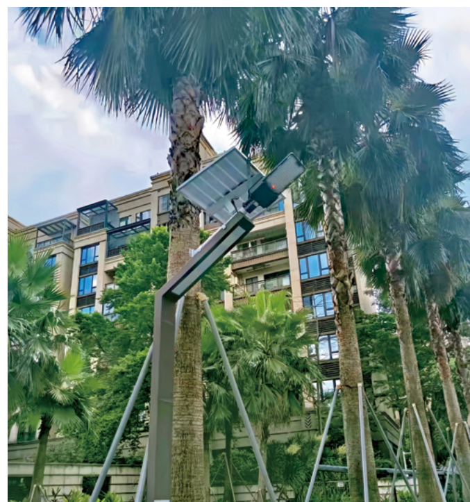
Photovoltaic Facility Installation for Park Street Lamps
