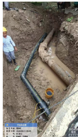
Figure. The site of gas pipeline network renovation conducted by Nantong Dazhong Gas
