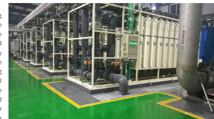
▲ Beidagou sewage treatment system of Angang Steel
