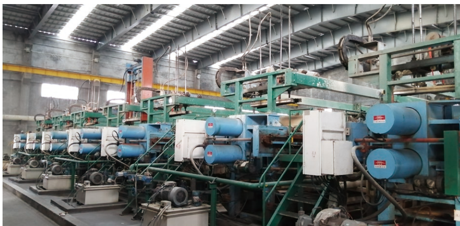
Sludge recycling equipment 污泥回收設備
