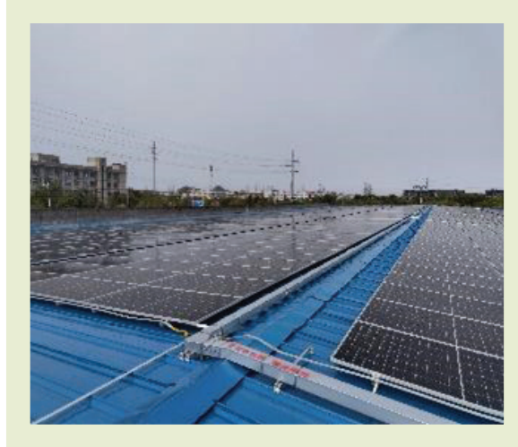
One of Hengan factory distributed photovoltaic power generation project 恒安工廠光伏發電項目之一
