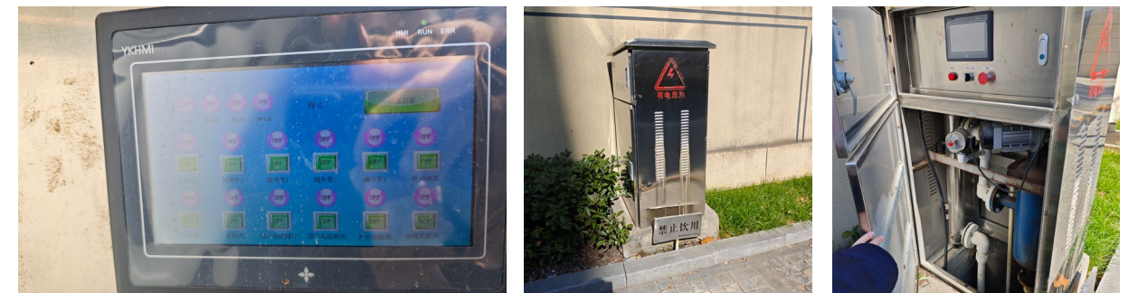
Rainwater Recycling at Deqing Company
