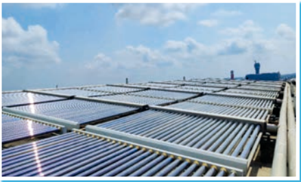
☀ Solar energy plus air source heat pump 太陽能加空氣源熱泵
