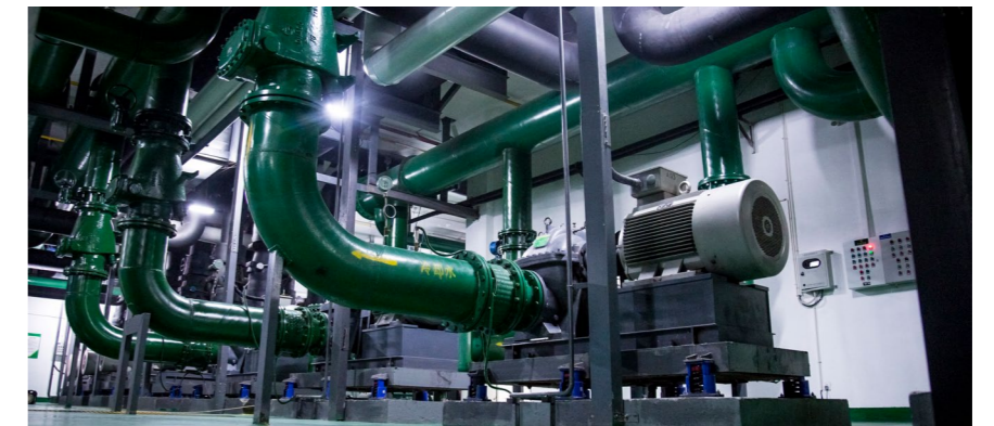
A low-carbon energy station of CEC Eastern Intelligence Valley
