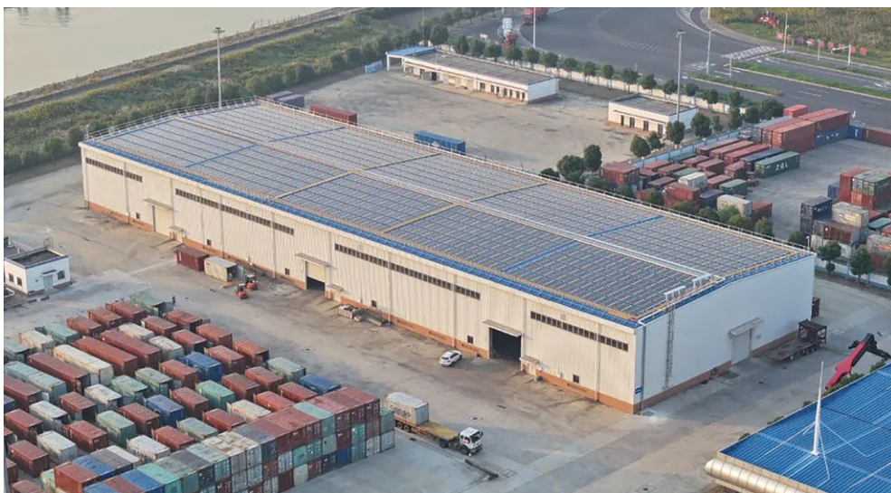
The distributed rooftop photovoltaic power station in Nantong Tonghai Terminal stated generating electricity since November 2023. It is estimated to generate more than 1.7 million kWh of clean electricity per year.
