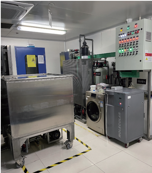
Animal rooms wastewater treatment facility
