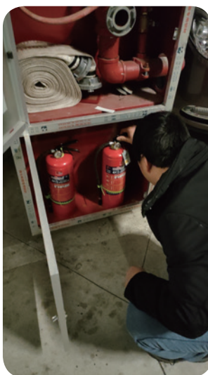
Regular Firefighting Equipment Inspection 消防器械定期檢查
