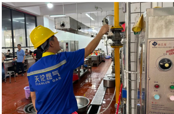
Chaozhou Company is carrying out a special campaign for the investigation and rectification of hidden dangers among users.
