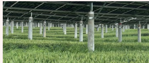
Hubei Xiangbei Agricultural-PV Complementary Project
