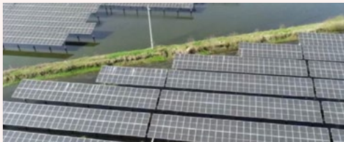
Hebei Nandagang Fishery-PV Complementary Project
