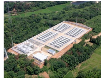
Xiangyin Project Liquid Cooling Energy Storage DC Cabinets
