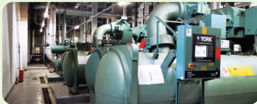
Figure: Converter upgrade project of YORK centrifugal unit
