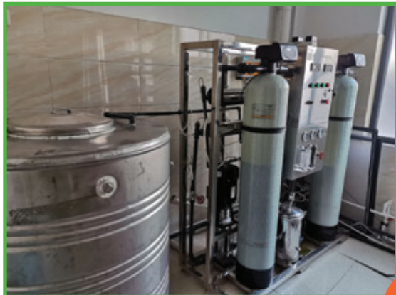
Water Purification Equipment
