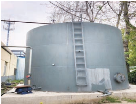
Steam Recycling System Installed
