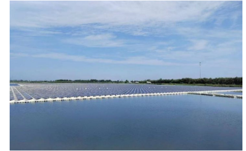
Peixian Hongyue Floating PV Power Station: The planned land use is entirely idle water surface from coal mining subsidence areas, achieving long-term protection of the aquatic environment.
