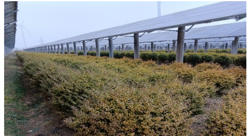
Xinyi Xinri Agri-PV Complementary Power Station: Planting greenery in the PV area improves land utilization. The pruning and management of greenery require a large number of people, thus local labor employment issues have been addressed.
