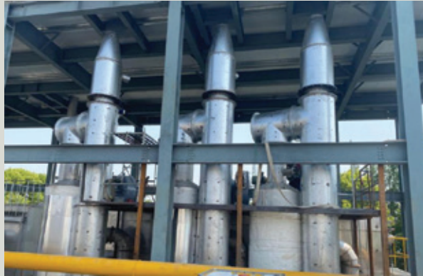
Exhaust Gas Purification System Field
