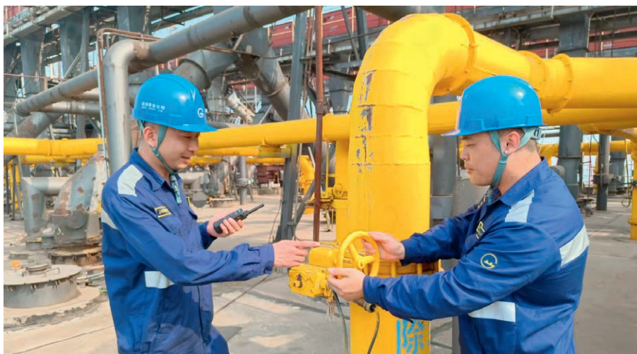
Maintenance staff of General Cargo Port Branch inspect silo dust collection system
