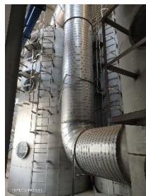
Spraying Tower for handling of paint exhaust
