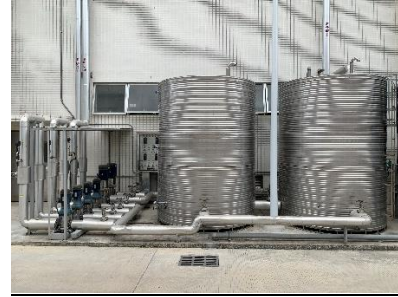
Heat Recovery Device
