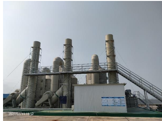
Acidic Mist Exhaust Treatment Facilities
