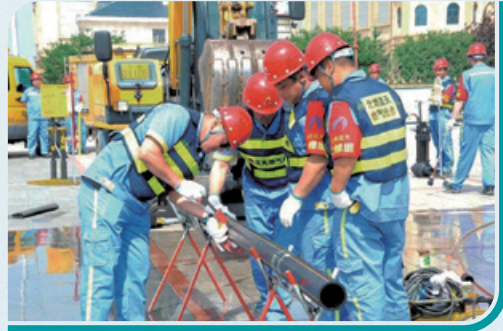
Emergency rescue drill for gas industry of Songyuan City and underground pipe network of Songyuan Beijing Gas Blue Sky conducted by Songyuan Beijing Gas Blue Sky New Energy Co., Ltd. (松原市北京燃氣藍天新能源有限公司) in 2023
