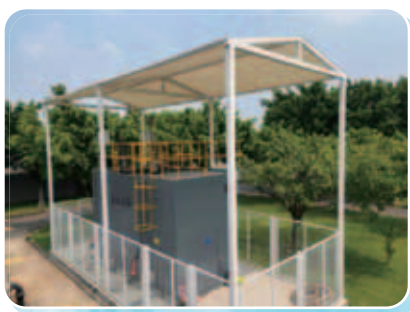
Integrated Facility for Aerobic Granular Sludge - Membrane Bioreactor
