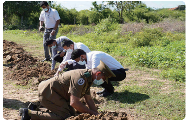
The District Secretariat and the Department of Wildlife Conservation work together to set up a fence to keep the elephants out.
