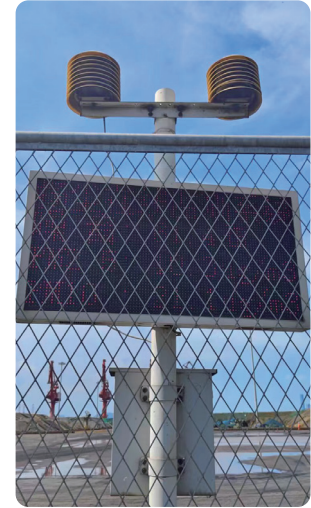
Four dust and noise monitoring devices installed along the perimeter of the Zhangzhou Port, with real-time data display.
