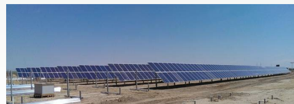
Ortalyk's PV power plant
