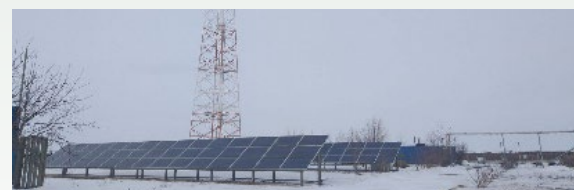
Semizbay-U's PV power plant
