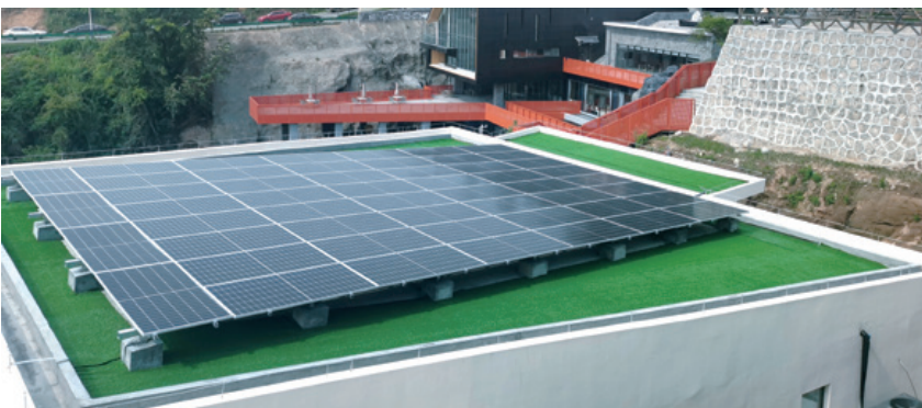
Rooftop PV of public buildings in CR Hope Town, Nanjiang
