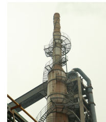
Mahong Plant's desulfurization tower
