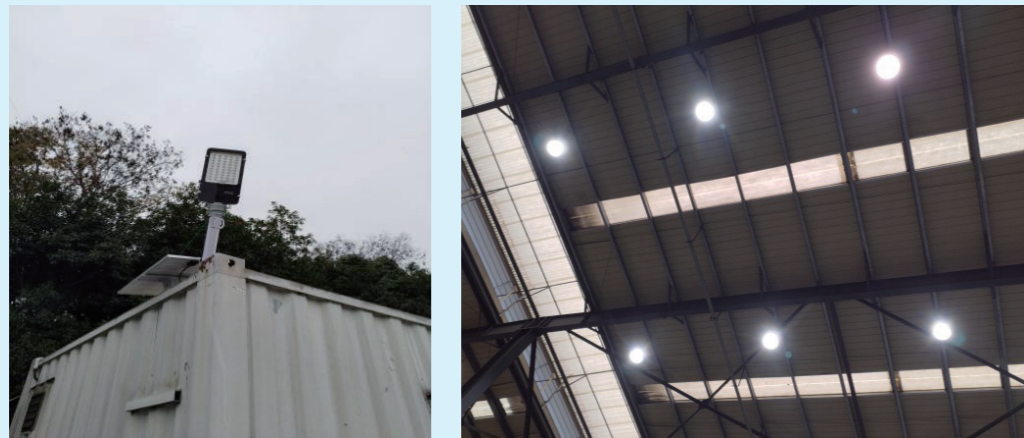
Installation of solar street lamps on the production base to reduce the power consumption
