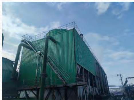
Replacement of high-efficiency square towers for thermoelectric cooling towers 熱電冷卻塔更換高效方塔
