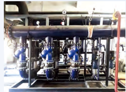
北京四環非供暖季空調熱水循環泵運行改善 Operation improvement of air-conditioning hot water circulation pump at Beijing Sihuan during non-heating season
