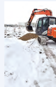
吉林匯康污水站工業水管線改造項目 Jilin Huikang sewage station industrial water pipeline renovation project
