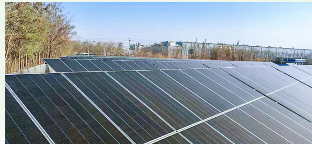
Distributed Photovoltaic at Tianjin Factory
