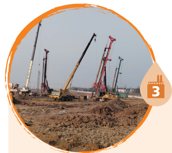
位於湖北荊門的溶劑廠房(在建中) The solvents plant in Jingmen, Hubei (under construction)
