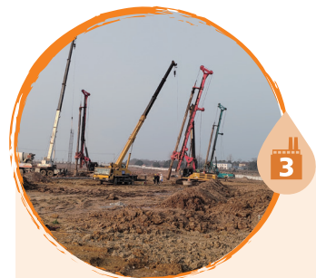
位於湖北荊門的溶劑廠房(在建中) The solvents plant in Jingmen, Hubei (under construction)
