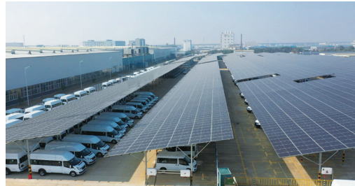
Nanchang Jiangling Photovoltaic Power Plant + Carport 南昌江鈴光伏電站+車棚
