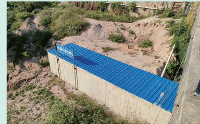
Zhaoqing Kangzhou Port leveraged a rainwater collection system within the terminal to collect water for reuse in landscaping or dust suppression, conserving water resources.
