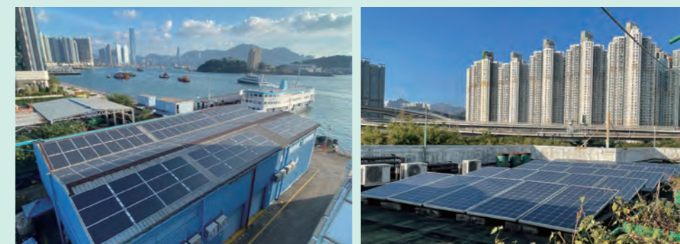
Sun Ferry installed a total of 323 solar panels with a total capacity of 109.85 kW that were distributed on the rooftops of the office building and two warehouses respectively. These solar panels collectively generate an average of 10,200 kWh of electricity per month, which are sold to China Electric Power Limited.
