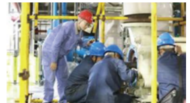
Jingxi Power Overhaul Site
