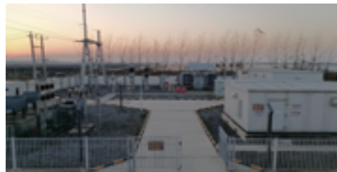
Substation of Jianli project
