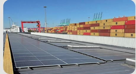
Tianjin Port Euroasia International Container Terminal Co., Ltd. Inspection Center Roof Photovoltaic Power Generation Project
