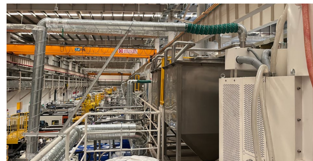
The Spray Tower and Biological Waste Gas Treatment Facilities at the Wuhan Stanley Molding Workshop.
