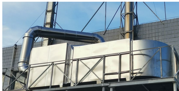
The Cyclone Tower and Bipolar Activated Carbon Adsorption Treatment Technology of Guangzhou Astemo Electrophoresis Workshop
