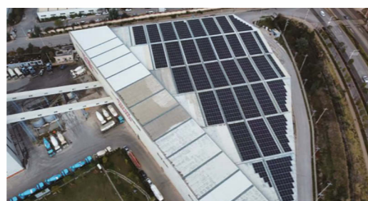
Rooftop distributed photovoltaic power station in Jingkai green production base- Phase II
