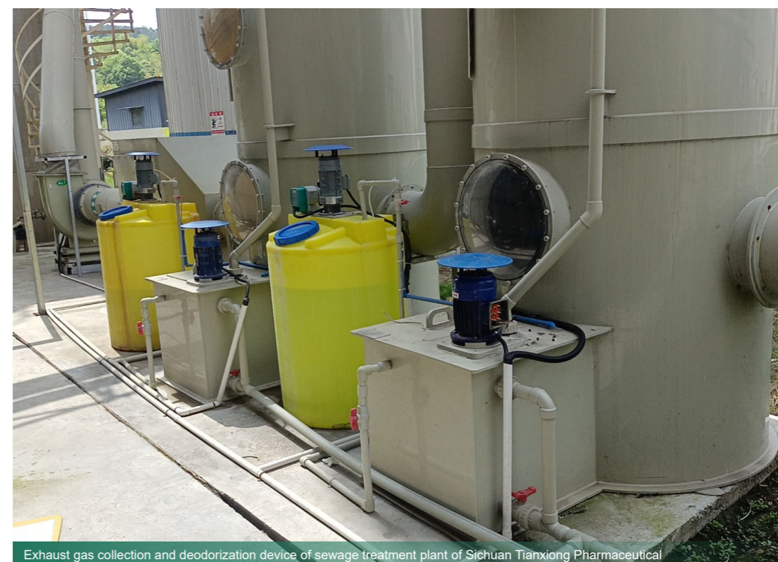
Exhaust gas collection and deodorization device of sewage treatment plant of Sichuan Tianxiong Pharmaceutical
