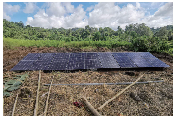
Solar powered water pump
