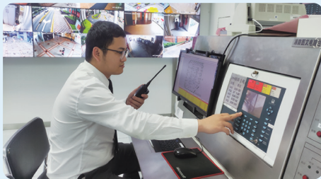
Victory Plaza | 24-hour intelligent fire safety monitoring
