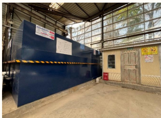
Sewage Treatment Stations
