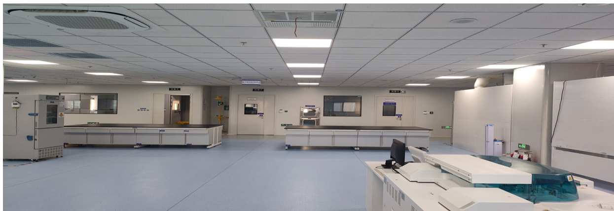
Labs Fully Utilizing LED Lighting and Variable Frequency Devices
