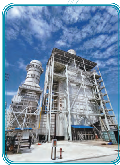
Waste heat boiler
