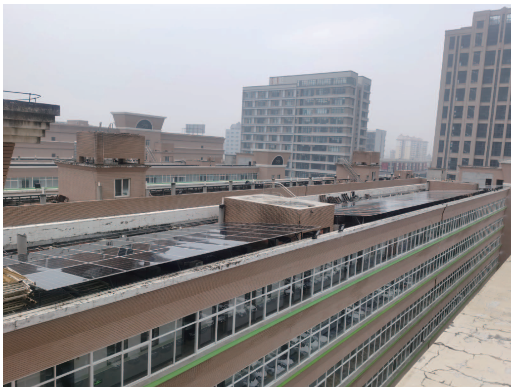
Photovoltaic power generation equipment
