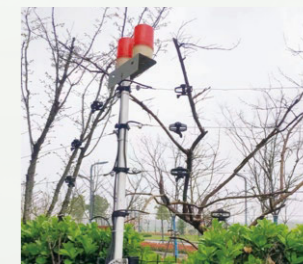
Perimeter protection alarm system
