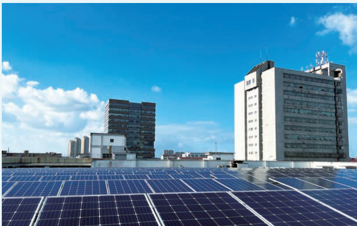
Industrial and Commercial Distributed Photovoltaic Power Generation Project of Suzhou Lvpu
